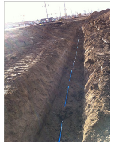
Wondering about the construction at SH52 and Frederick Way? It's a water line loop for the new 7-11! It will provide a second source of water supply for fire protection.
